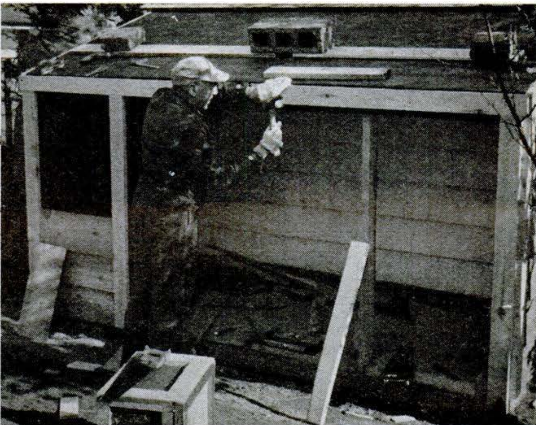
6 TAR PAPER is tacked to roof boards and side sheathing and secured under 1 1/4" by 4" finish strips. Weighted boards on roof keep paper from blowing loose.
